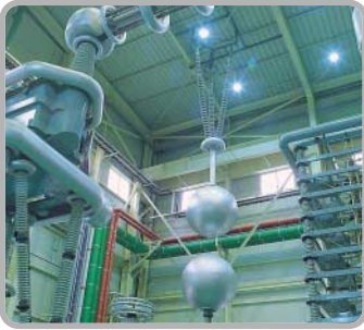
High Voltage Test / Impulse Test
